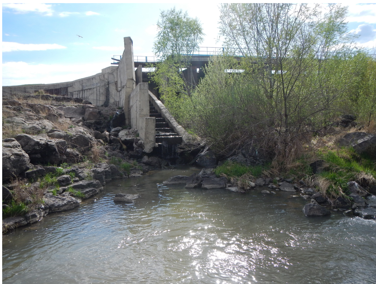
Fig. 4. Site N6 with fish corridors of a hydro-power station and a small lake.
